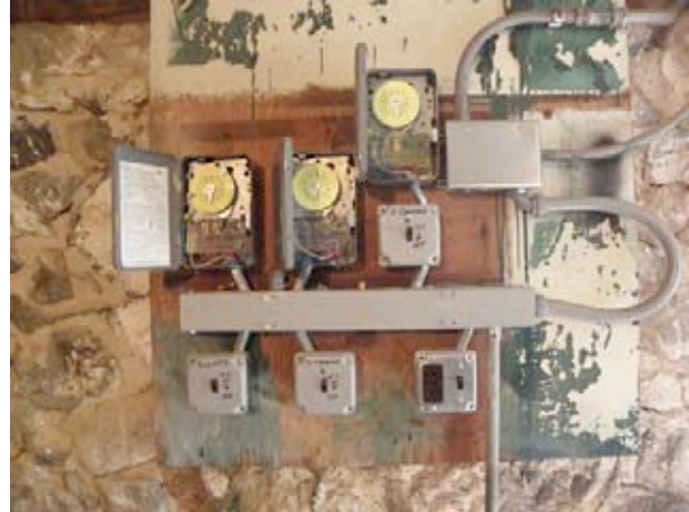
Detail of Electric Time Clocks & Switches Just Inside of Basement Doorway. (The Electric Panel is Located in the Adjoining Bath House.)
