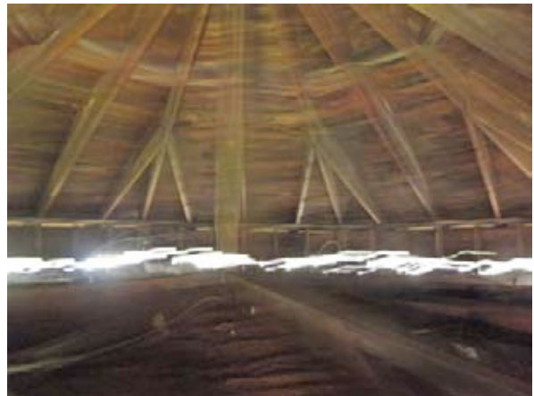
From the Ceiling Hatch Looking at the Center Post that Holds Up the Ceiling
