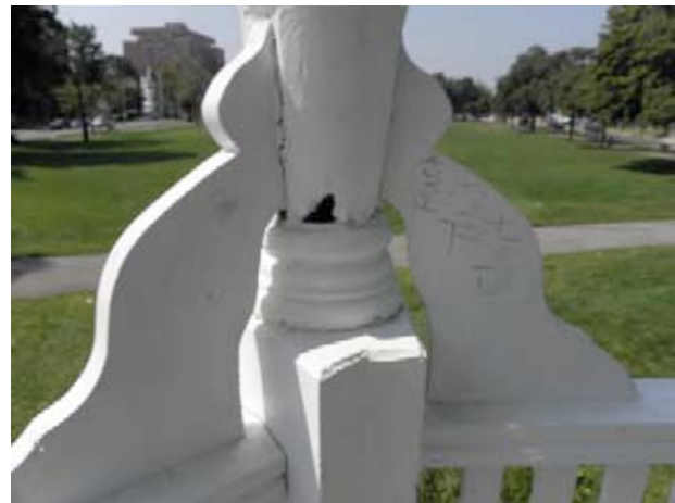
Column #4: Serious Rot at Base of Column
