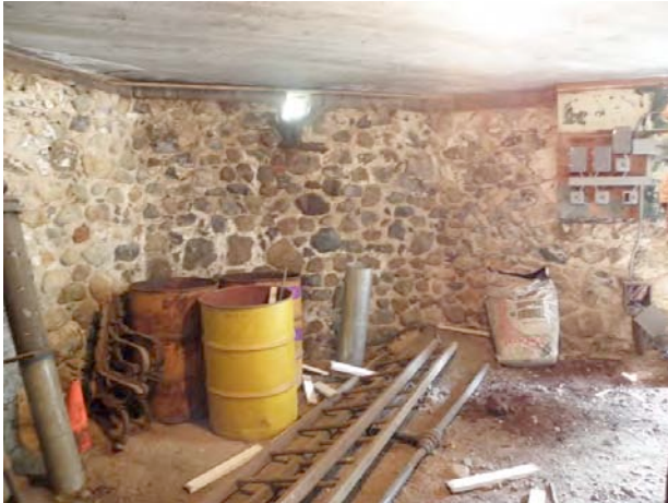
Basement View Showing Electric Underground Service Leading to the Electrical Backboard.
