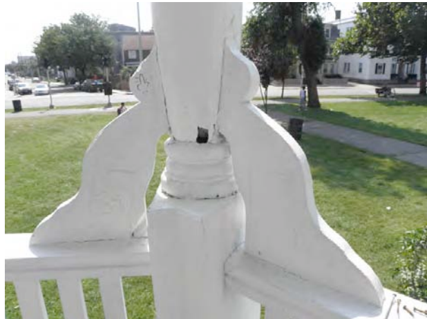
Column #3: Serious Rot at Base of Column
