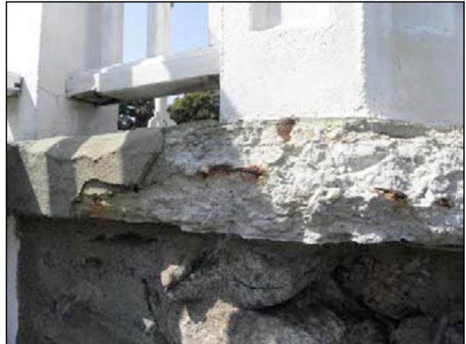
Detail of Deterioration of the Northeast Corner of Floor Slab
