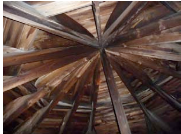
From the Ceiling Hatch Looking Up at the Center of the Roof
